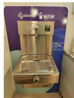
Reverse osmosis system installed in each working station
